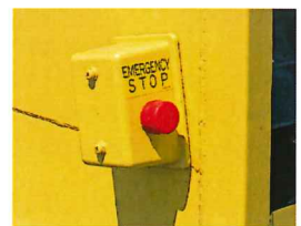
▲ Emergency stop control
